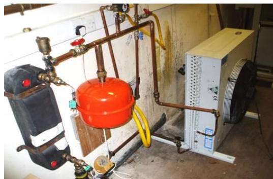
Figure 15. Shows the connections of the heat exchanger, water pump, heat rejection fan and expansion valve.
